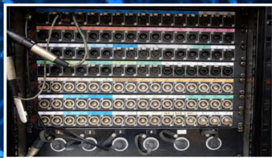
Ext. Termination Panel
